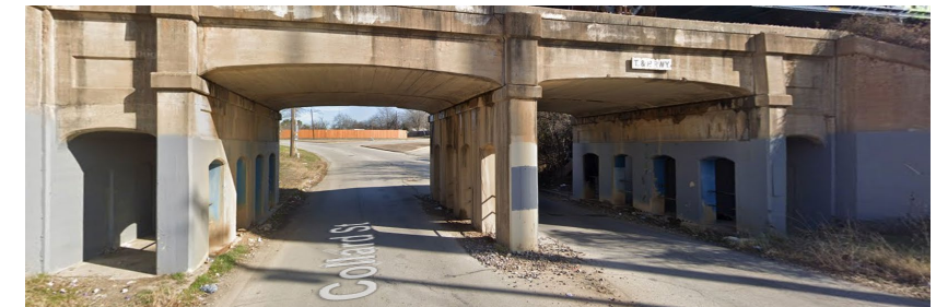
Existing cross-section and UP underpass and intersection along Collard St (images from Google Streetview)
