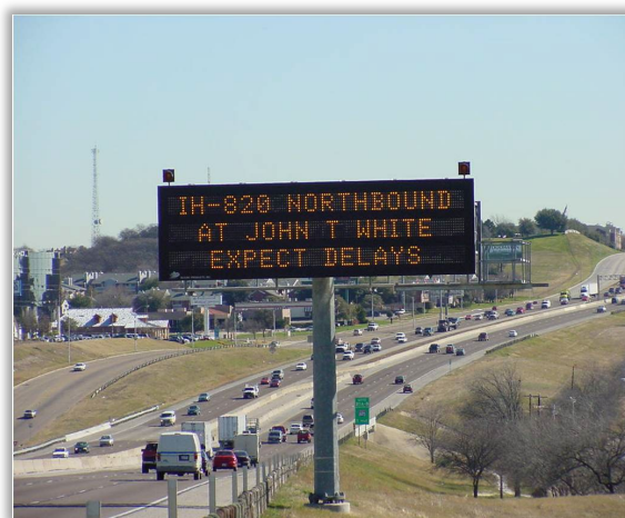
Dynamic Message Signs provide travel-time estimates and other information to improve commutes.
